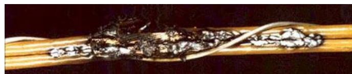
Figure 30: Example of arc tracking
